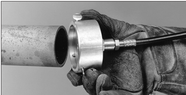
Figure 4.16 A welder prepares to install a backing dam over the end of a pipe to be welded.
